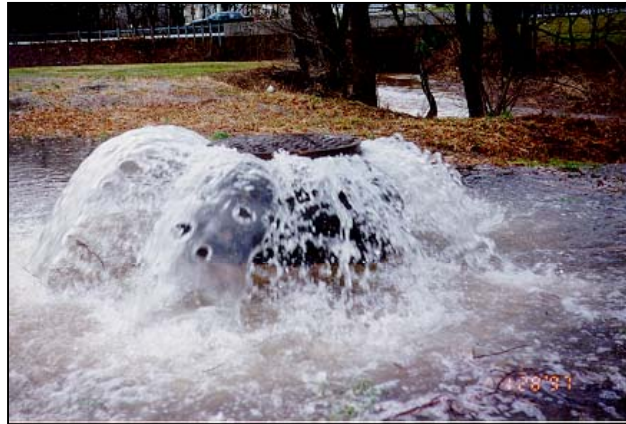
Figure 1.4.6-2 Overflowing Manhole Near a Stream
